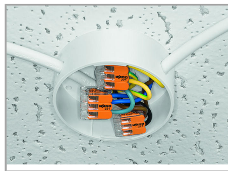
Lighting distribution in ceiling canopy
