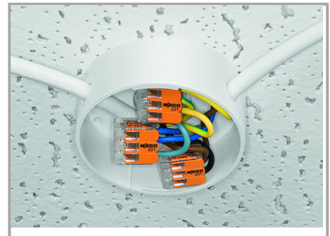
Lighting distribution in ceiling canopy
